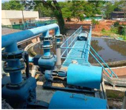
500 KLD STP at Kozhikode medical College
