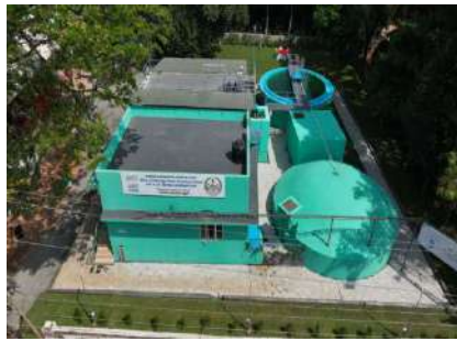
360 KLD STP at General Hospital, Thrissur
