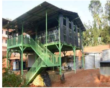
1 MLD STP at Kozhikode medical College
