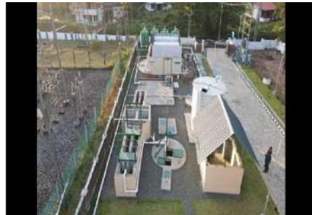
1 MLD CSTP at Padanappalam, Kannur
